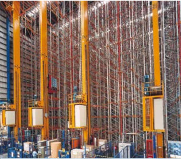
High Rise Storage Automated storage and retrieval
